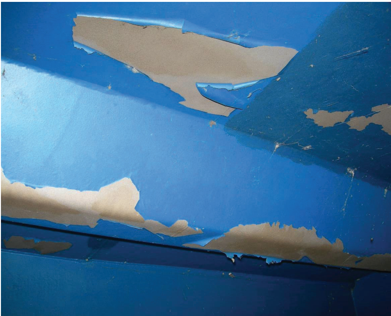
Figure 14: Damage to a bridge abutment with delamination of a blue polyurethane coating (photograph: German Federal Highway Research Institute).
